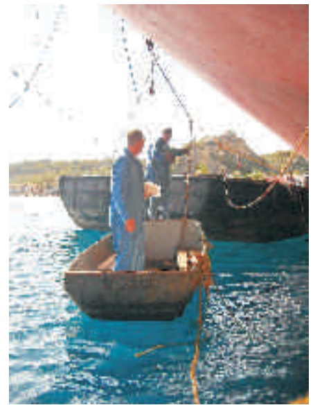
Welder Jason Cooper (front) and Daniel Haakinson (rear) using the "ferry" to get on land. This picture is taken from the cofferdam, where the welders were working. They are using the boat to get on the float and on land.
